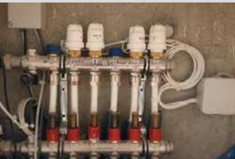
Raccordement des thermostats © R. Jobin
